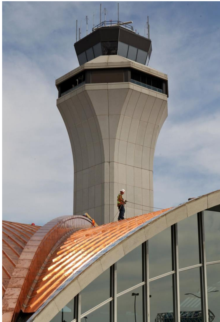
A worker stands on the last section of copper to be placed on the roof of Terminal One on Monday afternoon, Oct. 27, 2014, at Lambert-St. Louis International Airport. Photo by J.B. Forbes, jforbes@post-dispatch.com
